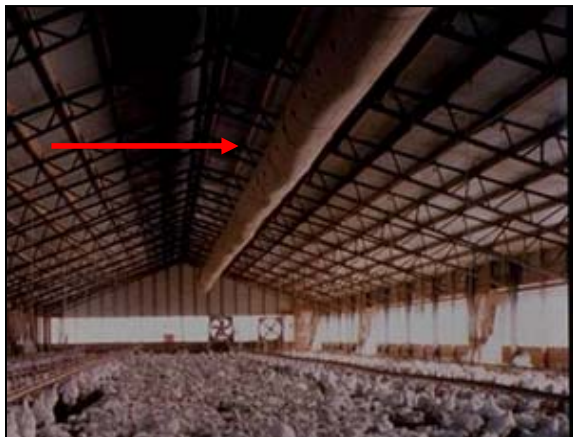
Figure 42: Plastic tube hot air distribution system used at the UA facility
