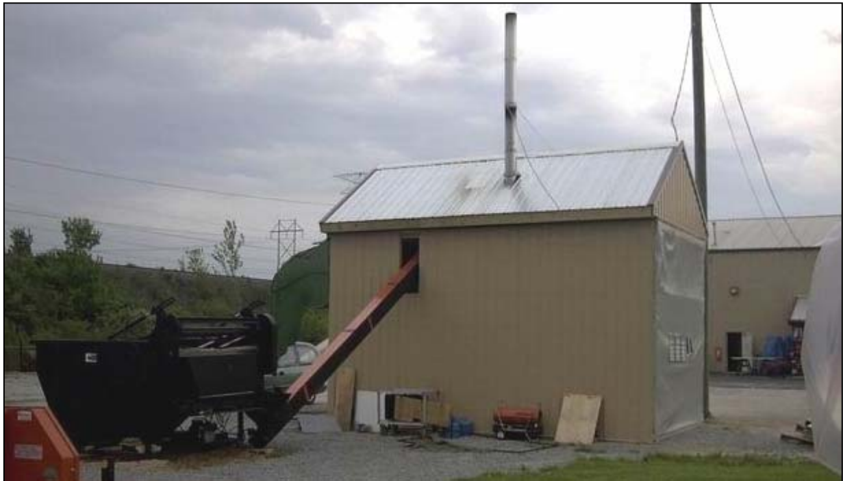
Figure A.4.6: Complete system with feed bin, belt conveyor, and furnace system (inside shed)
