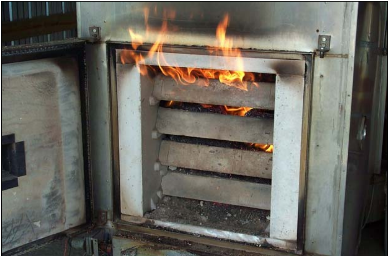
Figure A.2.6: Close-up of ceramic grate section
