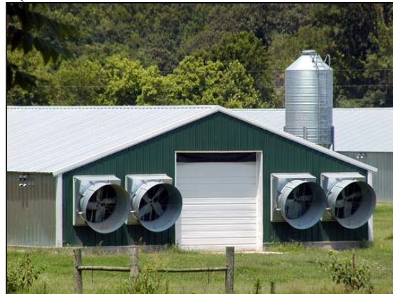
Figure 18: 48" exhaust fans on a newer style tunnel ventilated house (this house has 4 exhaust fans at each end)
