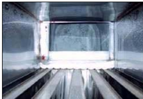
Figure A.4.3: Inside view of air-to-air heat exchanger (foreground) and heat deflector shield (background)
