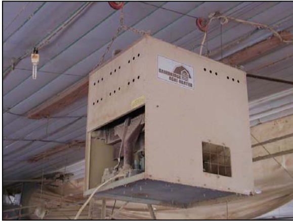
Figure 25: 120,000 Btu forced air heater (suspended from the ceiling)
