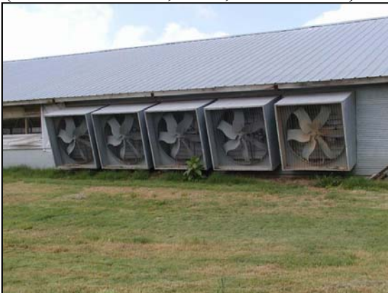
Figure 17: 48" exhaust fans on an older style tunnel ventilated house (this house has 10, not 8, exhaust fans)
