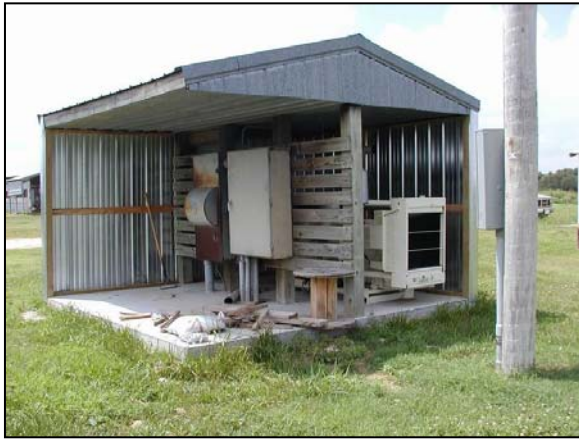
Figure 19: On-site electric generator & shed
