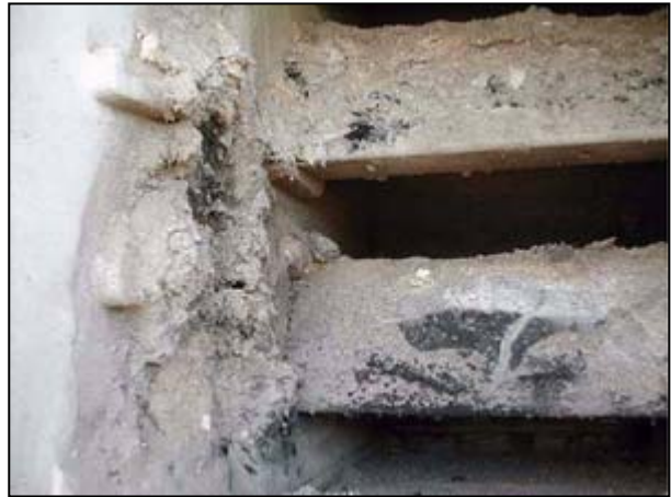
Figure A.3.10: Slagging from litter testing
