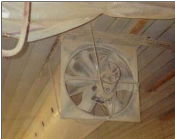
Figure 43: Axial fan that inflates the hot air distribution tube
