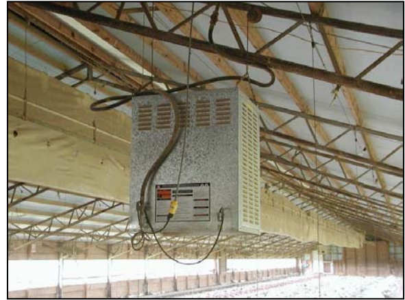
Figure 26: 240,000 Btu forced air heater (suspended from the ceiling)
